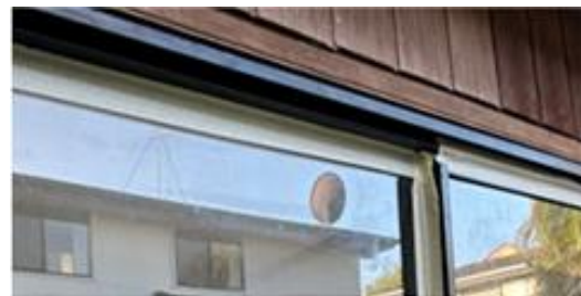
Figure 2. Sealed sliding doors
