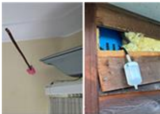
Figure 5. Air make-up point
