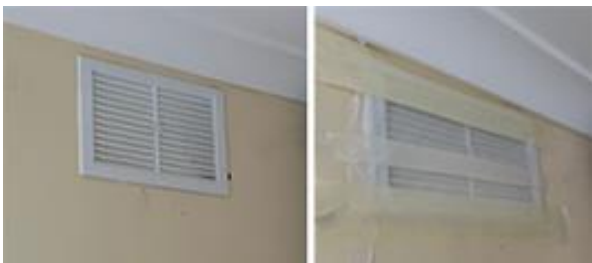
Figure 2. Wall vent: (a) original, (b) sealed
